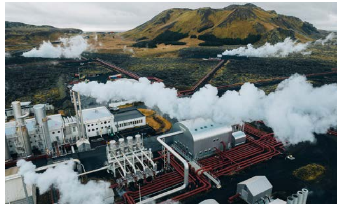
Two of Iceland's five largest geothermal plants are owned and operated by HS Orka
